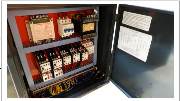
Detail showing electrical cabinet, with disconnect and fuse holders.
